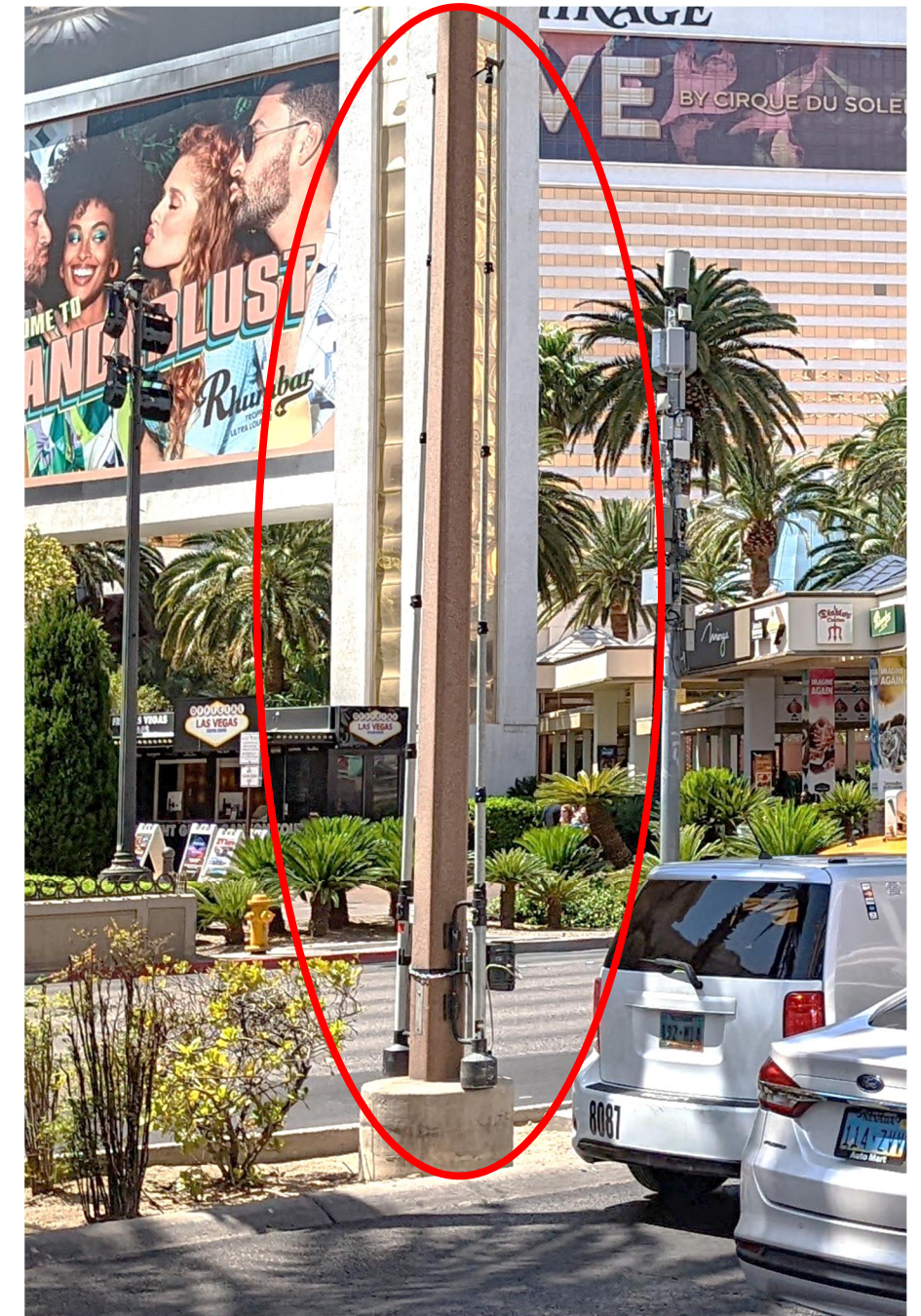
Photo 3.3 – Typical Installation of Camera to Collect Vehicle Volume Counts
